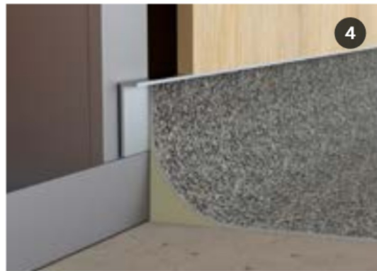
Raised vinyl floor
