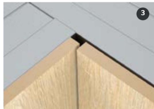
Open joint in internal corner
